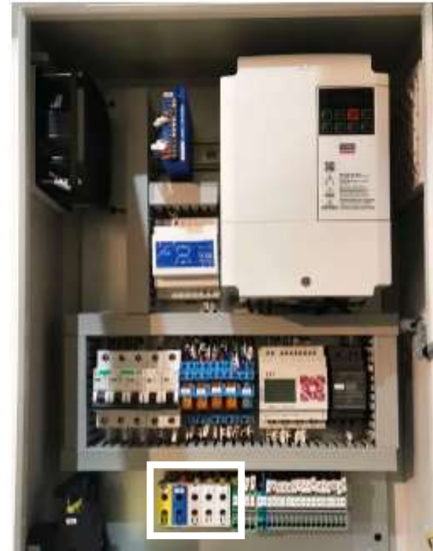
3 Phase + N + Ground power output on drive
