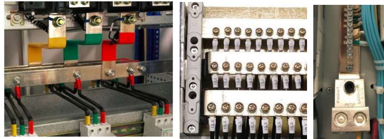
PANELS / MACHINERY / HVAC
